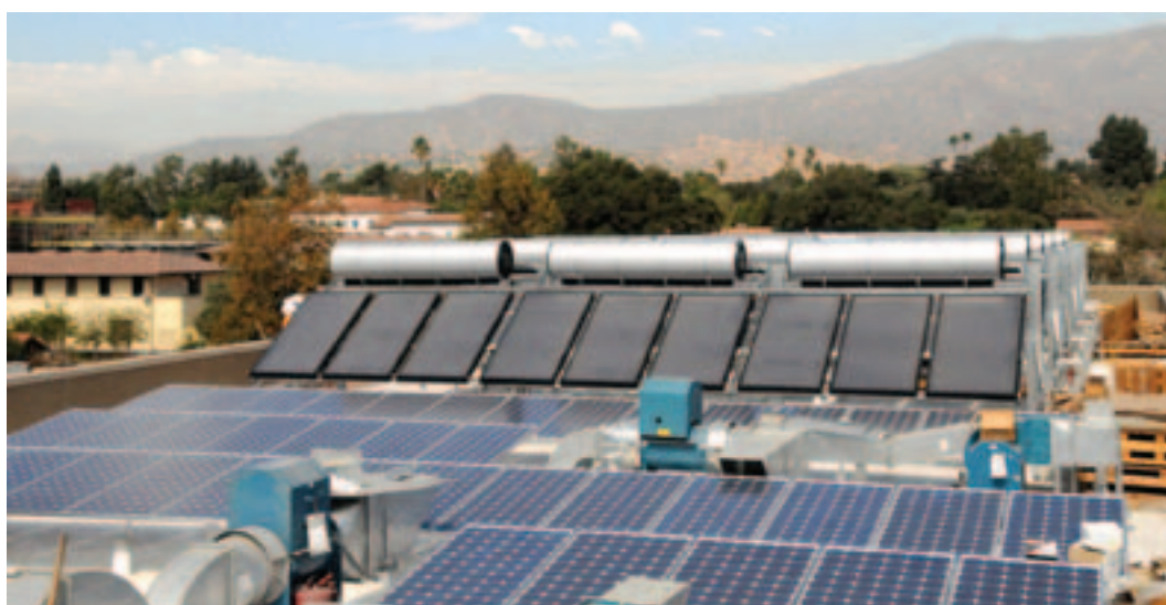
Photo 4.7 An installation of solar PV and thermal collectors on the same roof
