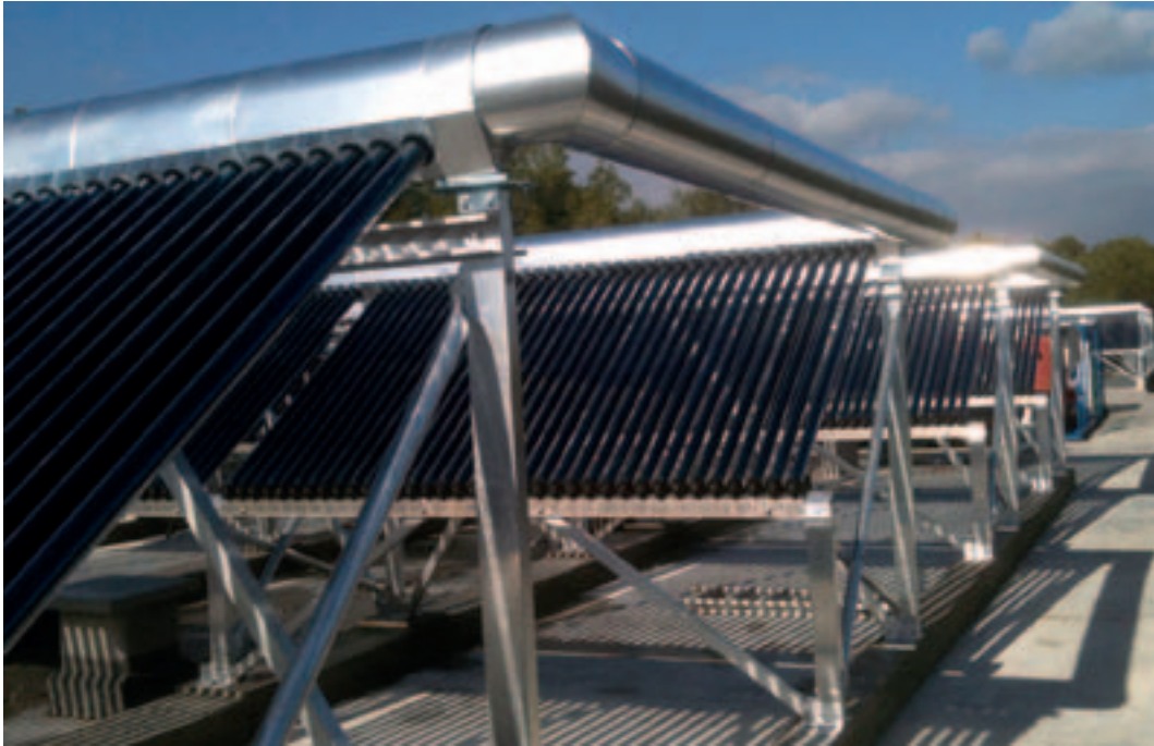
Photo 8.6 Experimental generation of electricity from non-concentrating evacuated tubes
