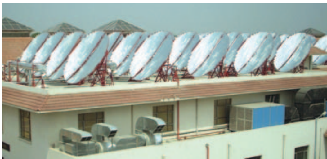
Photo 4.6 Solar steam cooking system at Shiridi for 20 000 meals
