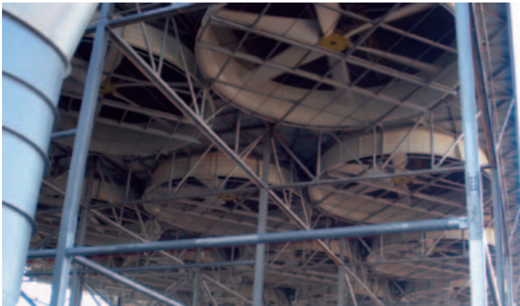
Photo 8.3 Dry cooling of the integrated solar combined cycle plant at Ain Beni Mathar, Morocco
